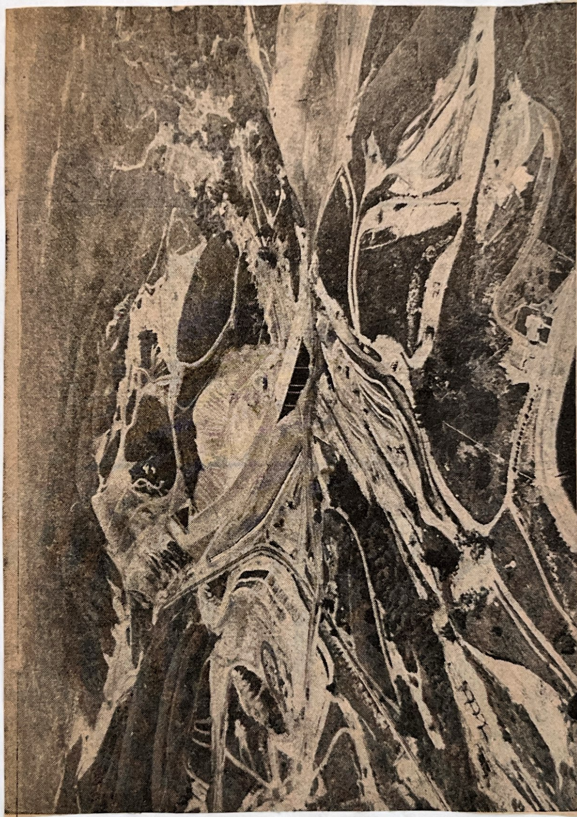
RESHAPING OF CANYON—Aerial photo shows how face of Brea Canyon is changing as segment of Orange Freeway is being constructed.
