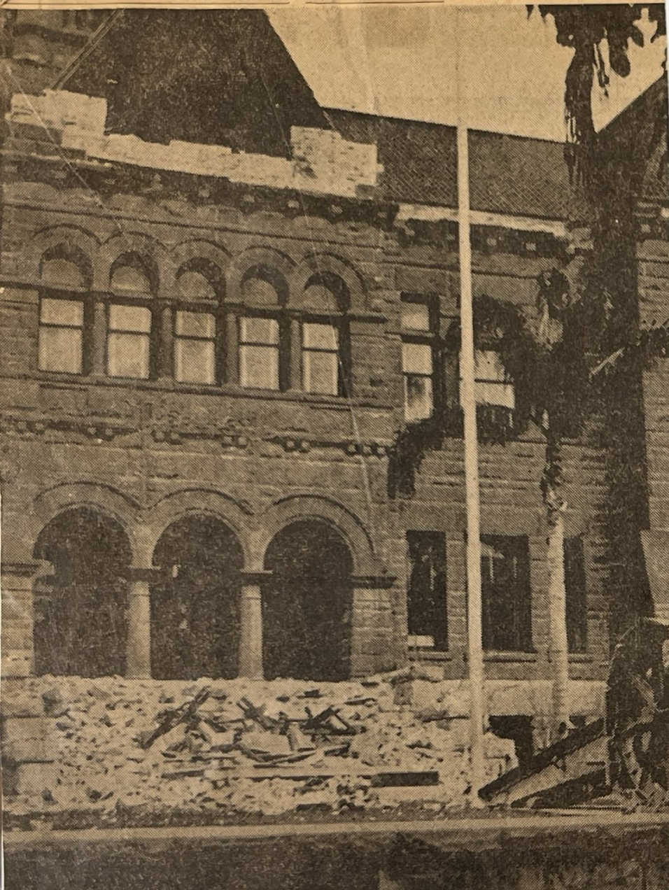
NO BUSINESS AT THE COURTHOUSE —The south entrance to the courthouse looked like this the day after the big quake. Other entrances to the building were also blocked off by debris. Succeeding temblors forced suspension of activities at the courthouse for several days. (Register photo)
