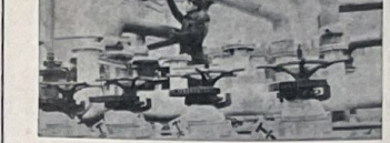
A scissor-like "jumper line" at a refinery pipe junction unit.
