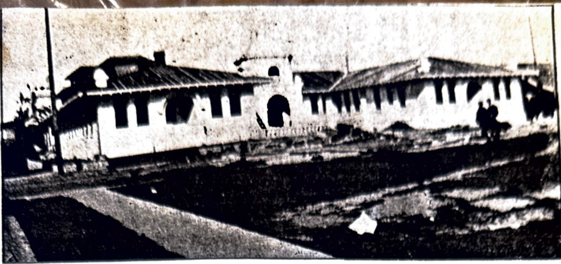
FULLERTON GENERAL HOSPITAL BUILDING BEING CONSTRUCTED Old facility, circa 1920, was operated by sisters from 1931 to 1953
