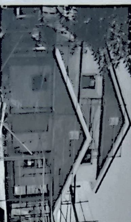
Now under construction by Habitat for Humanity at 101 S. Haver, this five-bedroom home is being built using alternative materials.
