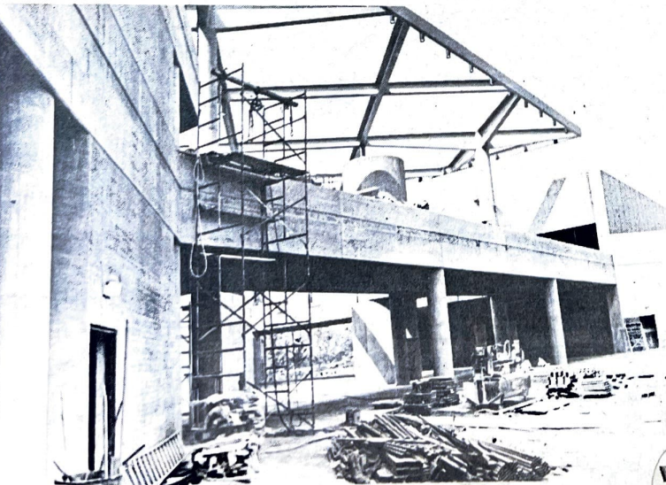
HARD HAT AREA..... The gallery is open but the public is not allowed in construction area.
