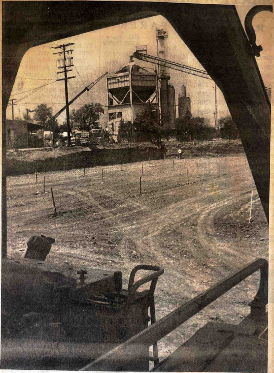
PROGRESS CONTINUES — An old familiar landmark in Brea, background, will soon be torn down to make room for redevelopment. In the foreground grading has been completed and staking is in place for a new senior citizen complex to be built on a site near Kirkhill Rubber Co.
