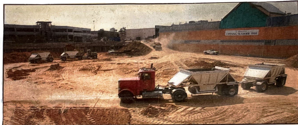
Construction is continuing on the exterior of Brea Mall as part of the shopping center's makeover.
