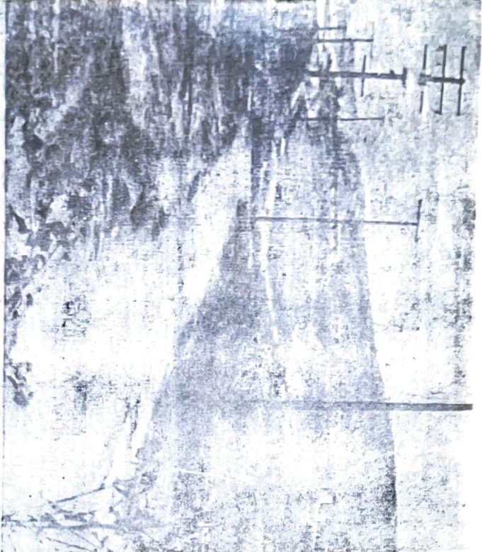
BASTANCHURY EXTENSION — One of the obstacles slowing traffic on Brea Blvd. is the $366,000 Bastanchury Road extension to State College Blvd. now under construction. The road is being widened to 84 feet at the Brea Blvd. intersection and flagmen
