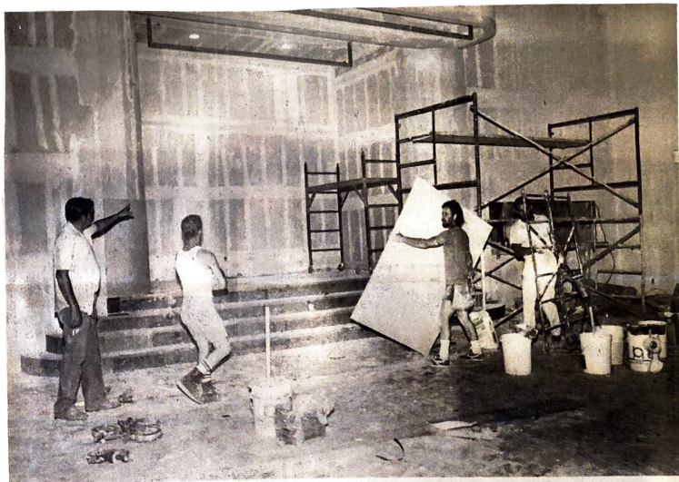
The finishing touches are added to Calvary Chapel of Brea's youth church and fellowship hall.
