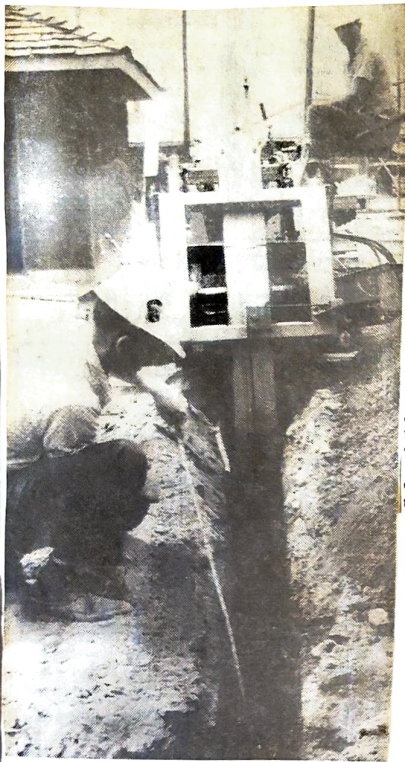
GOING UNDERGROUND — Construction Foreman Bob Todd measures three-foot depth of trench for buried telephone cable. Lineman Joe Trask operates new machine which digs at rate of eight-feet-per-minute, also does the "back-fill" job.
