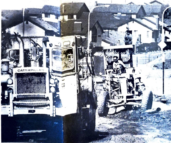
ROLL 'EM — County tractors begin the much-awaited extension of Lambert Road from Sunflower Street to Valencia Avenue. The road will, in effect, be connected to Carbon Canyon.
