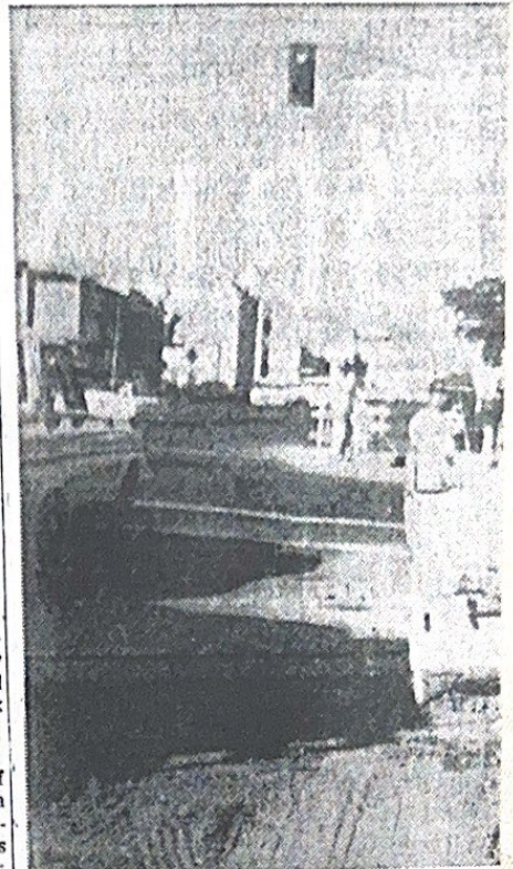
BREA BLVD. - IMPERIAL HWY. JO ic Telephone Co. is installing underg duits at Brea Blvd. and Imperial Hwy.
