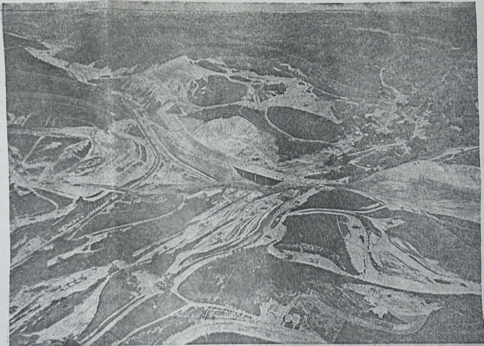
RESHAPING OF CANYON —Aerial photo shows how face of Brea Canyon is changing as segment of Orange Freeway is being constructed.
